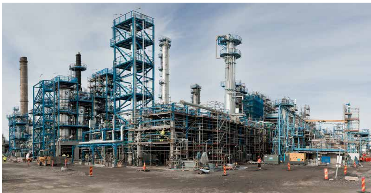
SCA's joint venture biorefinery in Gothenburg was commissioned in late 2023/early 2024.
