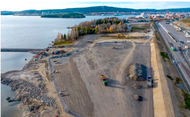
Logistics areas are growing behind SCA's new container quay, with an additional 30,000 square metres about to become available.
