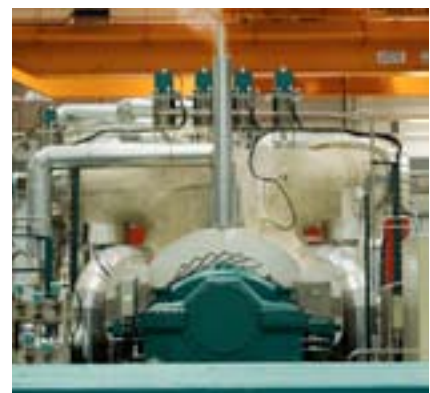
The new turbine in the Östrand pulp mill generates 0.5 TWh electricity per year and will improve SCA's energy balance.
